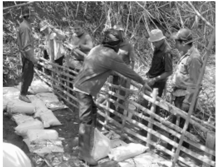
Conservation for better food production. Construction of a check dam in a community forest, Nam Jo village, Muang Phan District, Lampang Province, Thailand. (Photo: Jaruwat Kaewmahanin)
